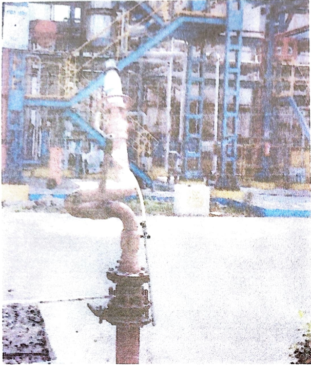
Annexure III – Picture of Fire Fighting:
