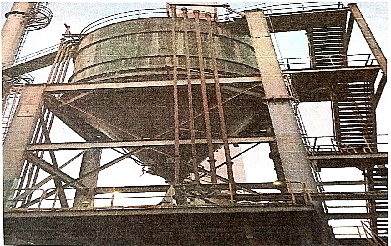
Annexure II – Picture of ash silo
